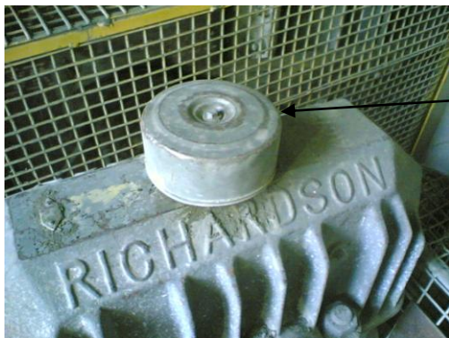
This breather looks OK from the outside.
